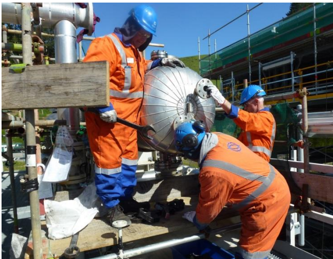
De-Ethaniser Condenser – Heat Exchanger Assembly
